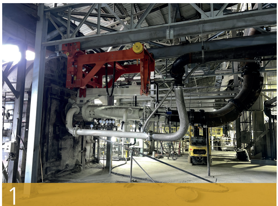
1. BURNER INSTALLED AT THE PRYOR PLANT KILN 1
